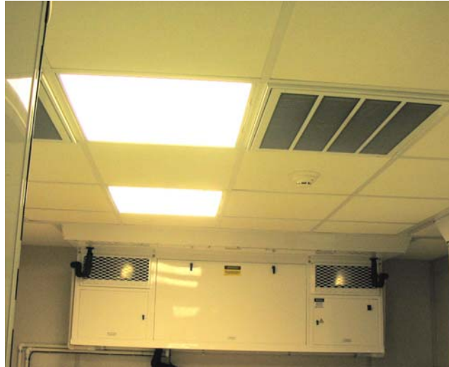
Figure 57: Equipment Room Lighting
