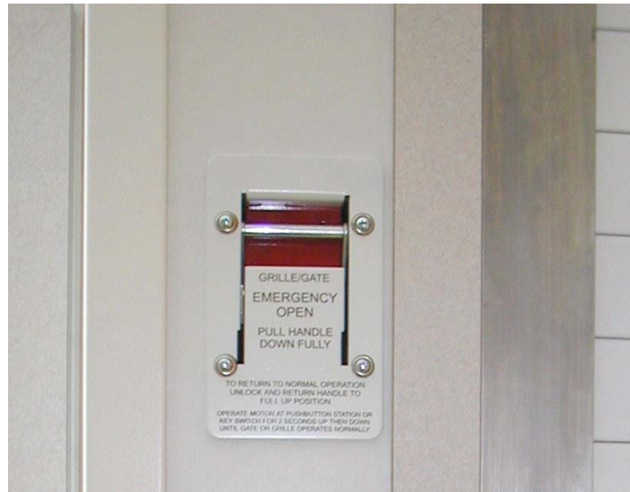
Figure 30: Roll Door Emergency Release
