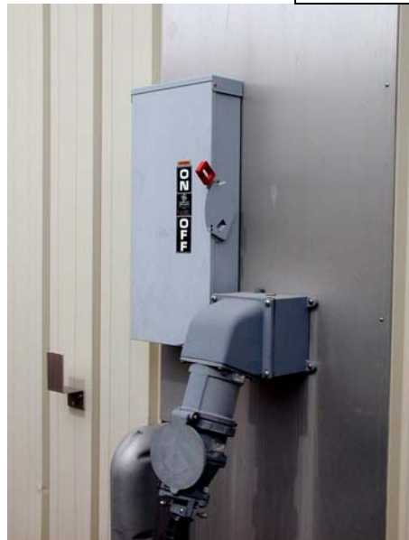
Figure 35: Shore Power Connection
