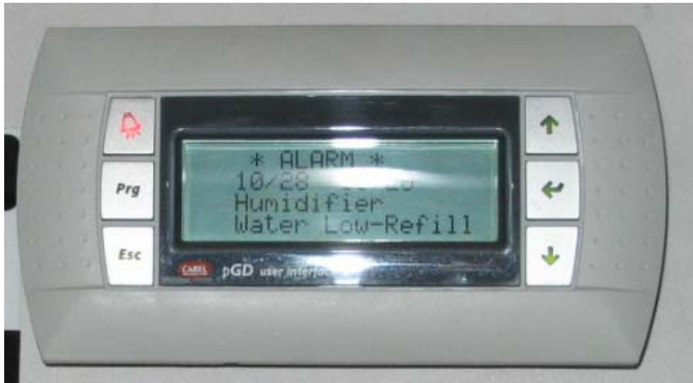
Figure 41: PDG Display A/C / Chiller Alarm Panel
