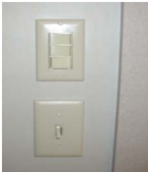
Scan Room Lighting
