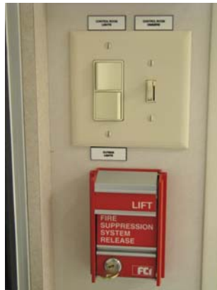
Control Room Lighting
