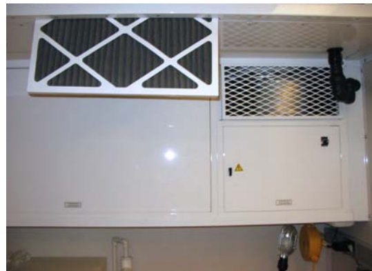
HVAC Filter Access
