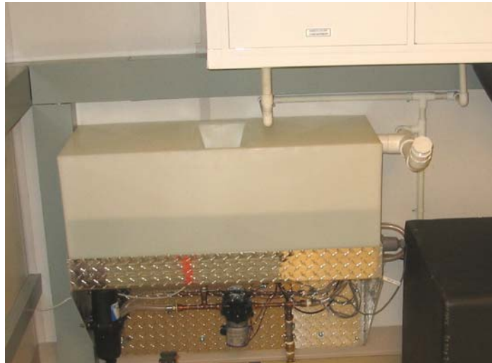
Figure 37: Humidifier and water supply tank
