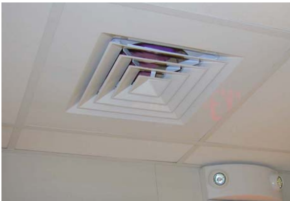
HVAC Vents Discharge
