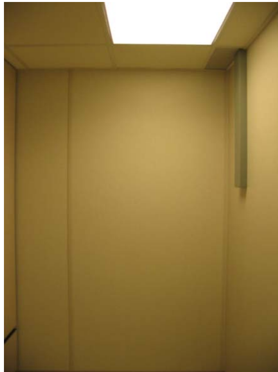
Figure 61: Changing Room Lighting
