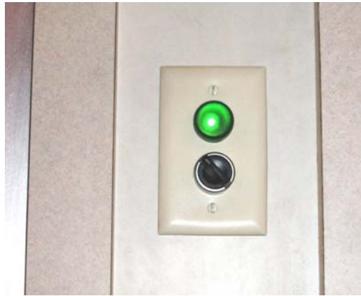
Figure 46: Platform Lift Power Switch
