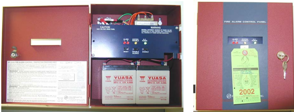
Figure 24: Fire Alarm Control Panel
