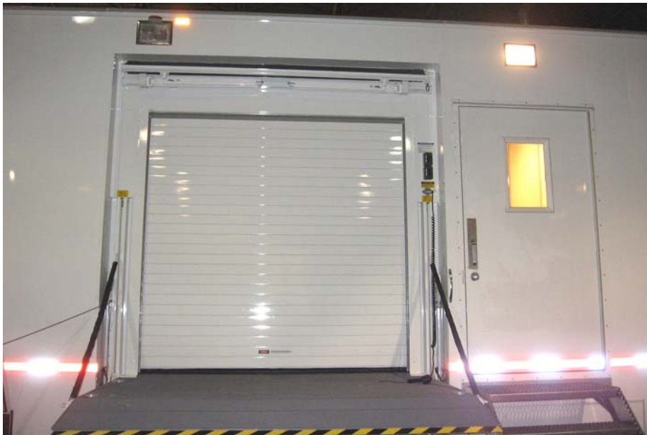
Figure 56: Staff Door Lighting
