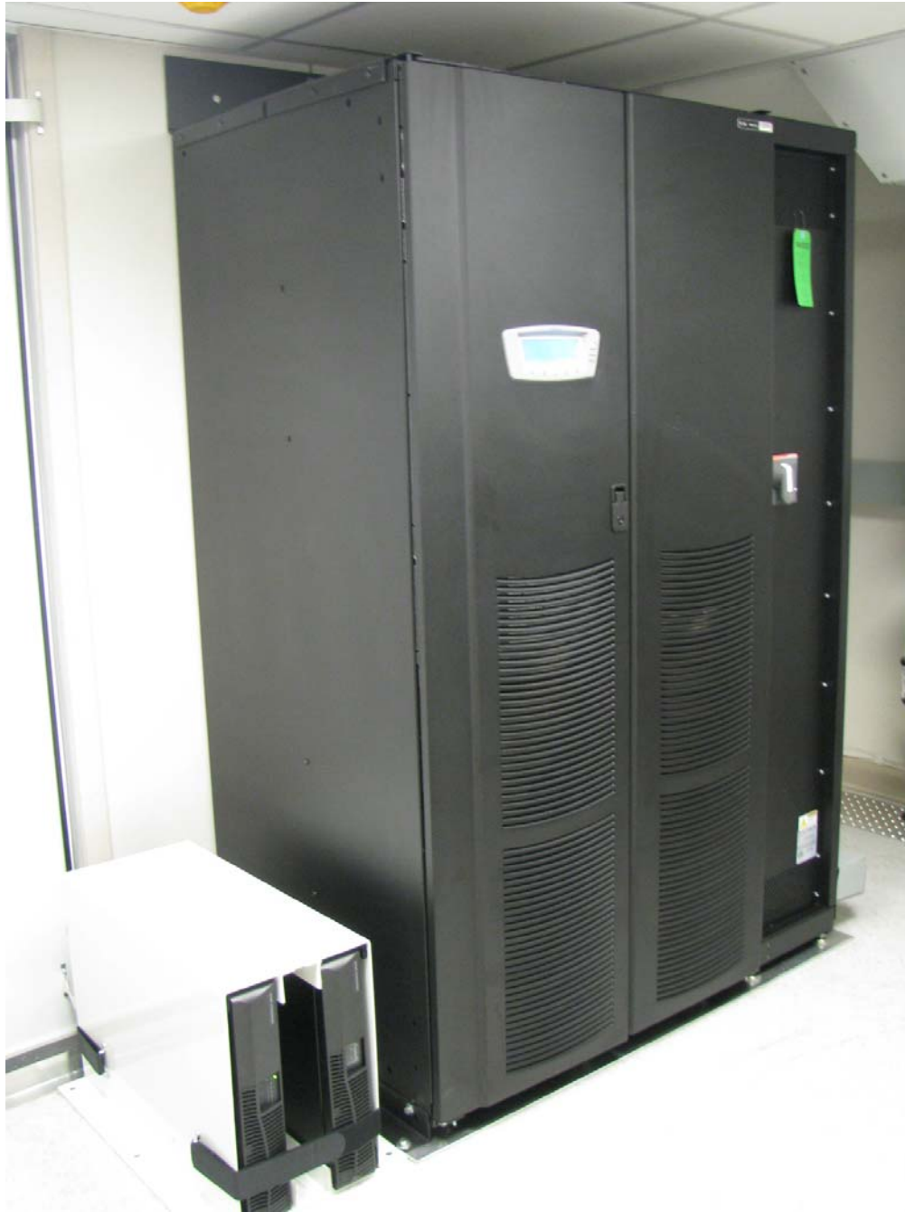
Figure 6: Equipment Room Overall
