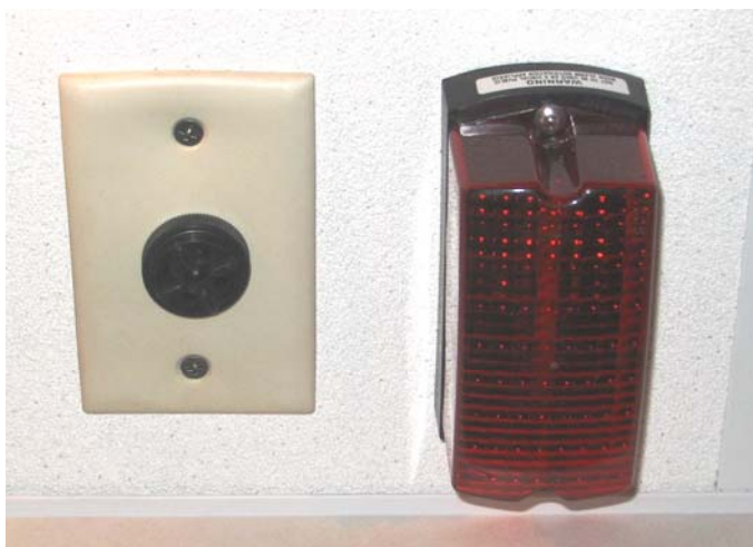
Figure 47: Platform Lift Strobe & Alarm
