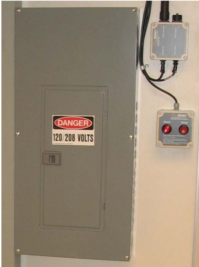
Figure 32: 120/208V AC Electrical Panel
