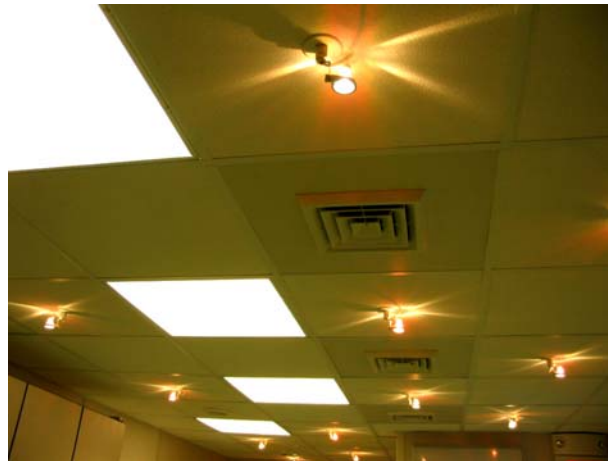
Figure 58: Control Room Lighting
