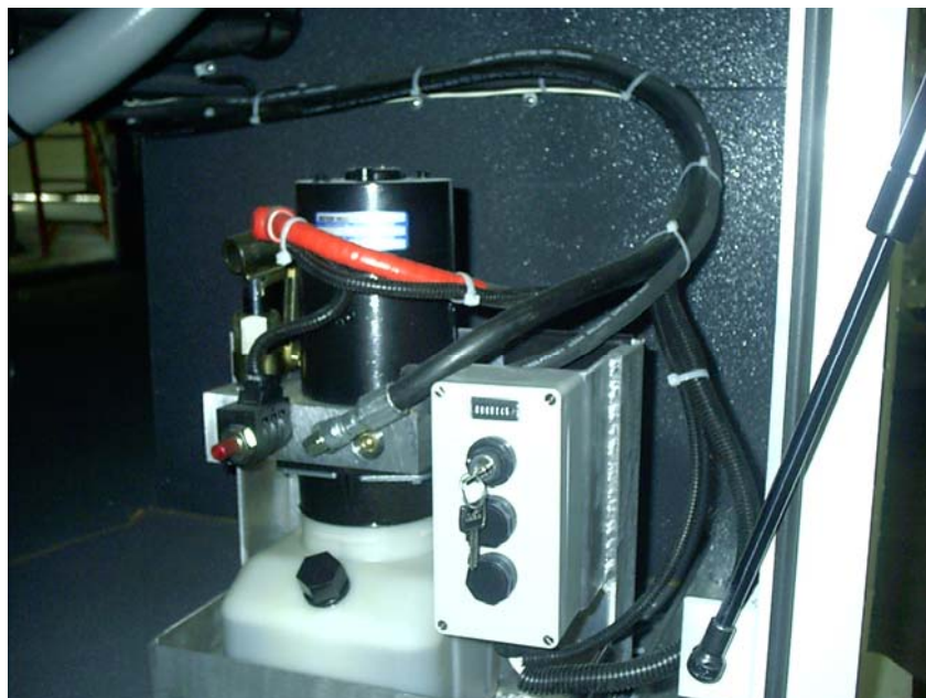
Figure 49: Platform Lift Service & Maintenance Controls
