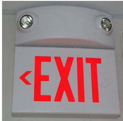
Figure 53: Emergency Dual Beam Lighting
