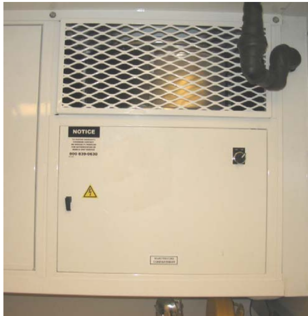
Figure 40: A/C / Chiller Control Panel
