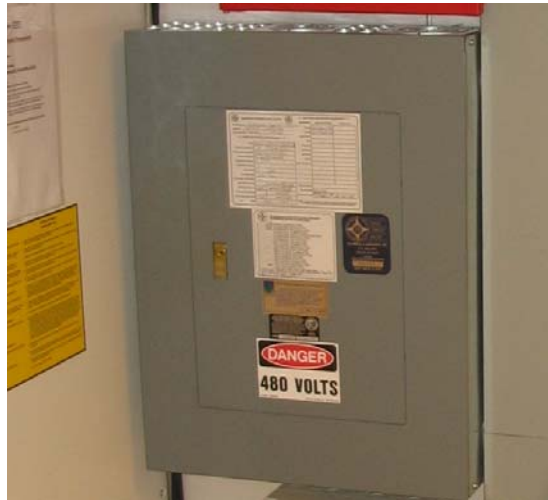
Figure 33: 480V AC Electrical Panel
