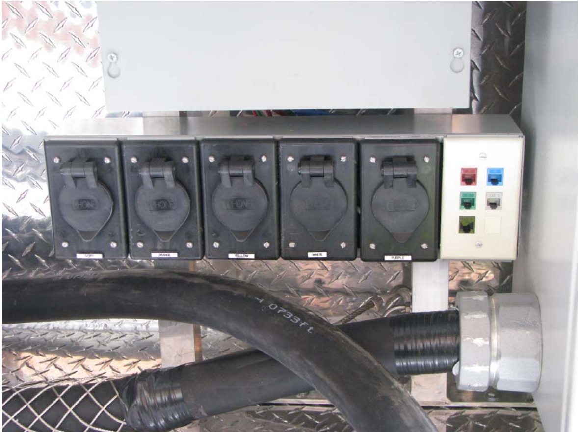
Figure 15: Phone & Data Line Connections
